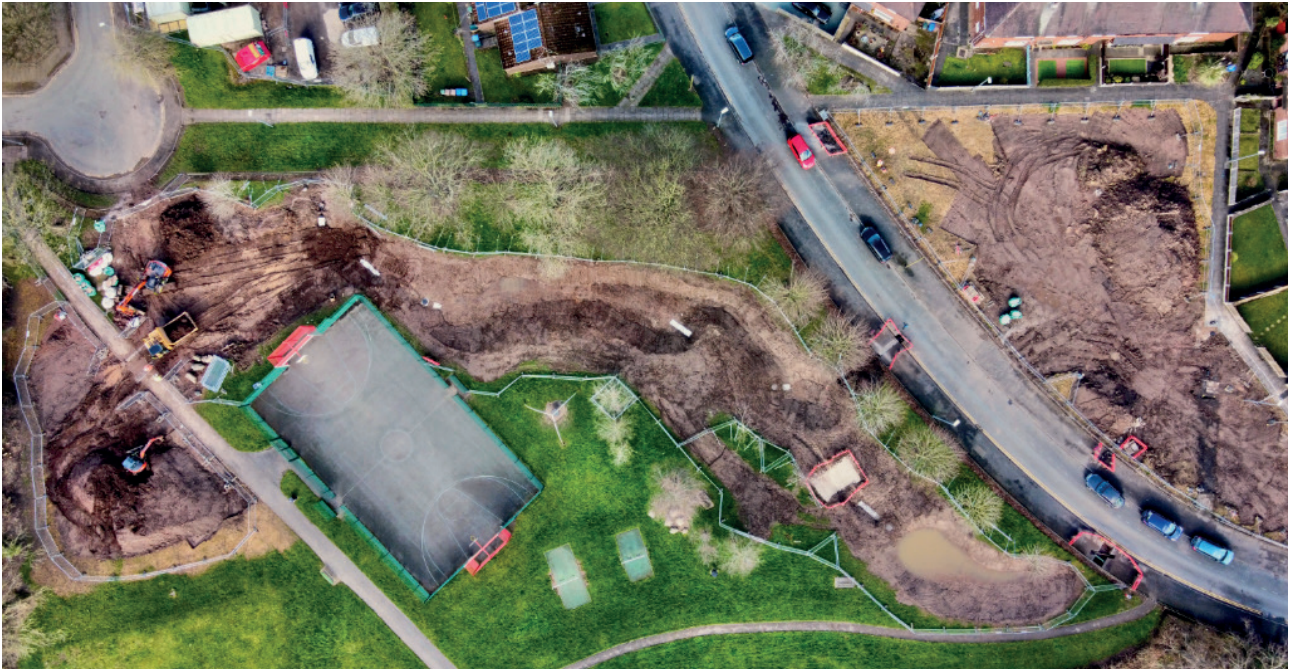
Figure 9. Birds Eye view of 2 of the 3 swales in the Hilton Road area of Stoke. February 2022 Note: Taken during construction, to indicate the scale of the SuDS being built
