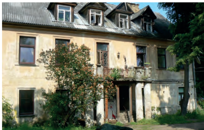
Dampness and rot in a C1900 multi-occupied building
