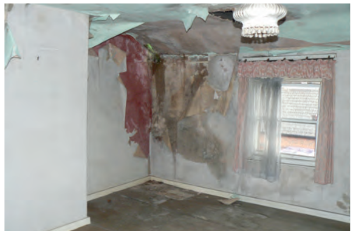
Dampness in a top floor bedroom of this house
