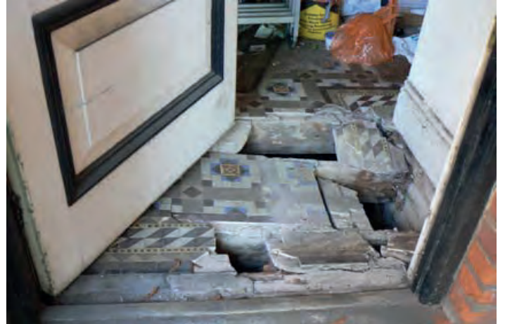
Rot in the floor of a c1910 semi-detached house
