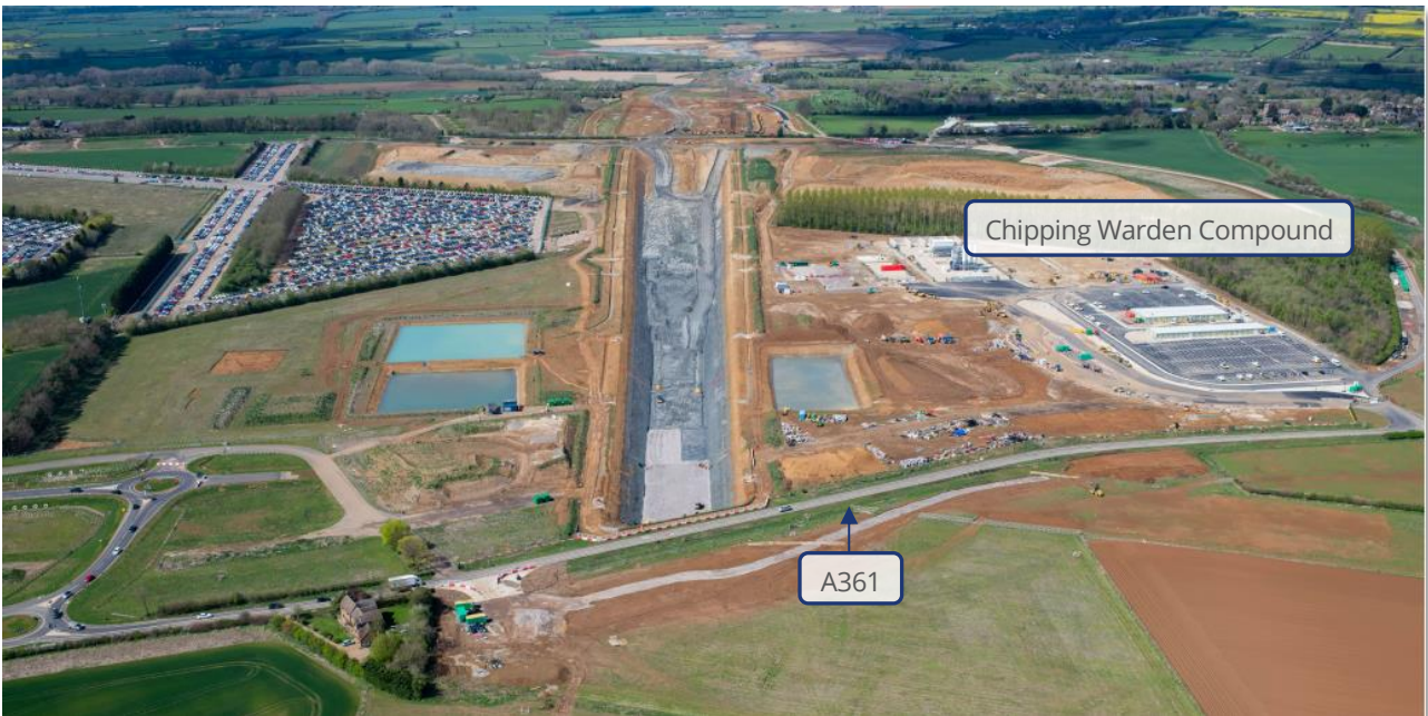
Figure 3: The above image is an aerial photograph, looking across the A361 from the East, showing our preparatory works for the Chipping Warden Green Tunnel, April 2022.
